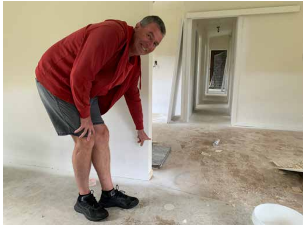
YMCA Camp Adair manager Dave Lockwood points to the level of floodwaters in the camp's staff accommodation during cyclone Gabrielle.
