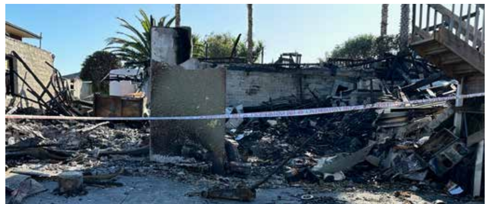
The Quinn’s home on Maraetai Drive was gutted by the fire.
