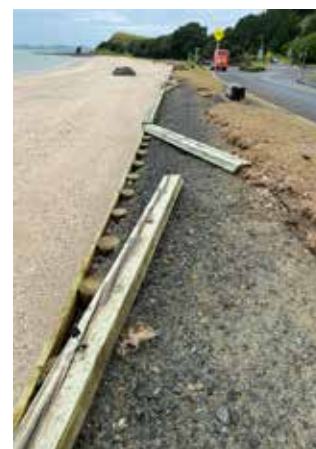
Right: damage to the Maraetai Beach seawall.
